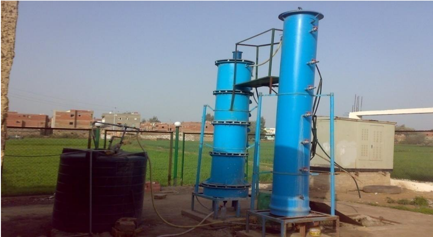
Pilot-scale combination of hybrid UASB reactor and Hanging Sponge (DHS) system treating domestic wastewater at experimental area (Mit Dafer village)
